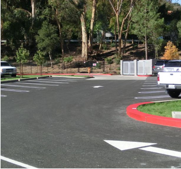
Figure 6-24. Porous asphalt collects and infiltrates runoff in the parking lot. (Credit: EOA)
