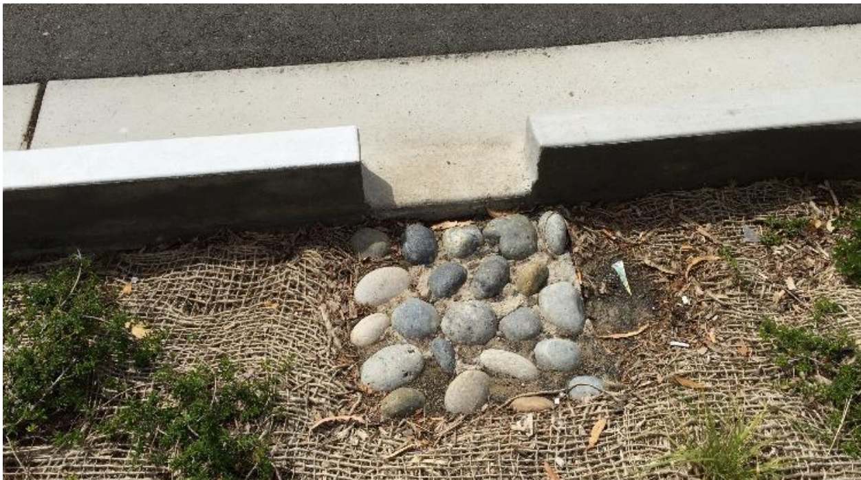
Figure 3-62. Jute netting holding soil and mulch in place in San Mateo. (Credit: EOA)
