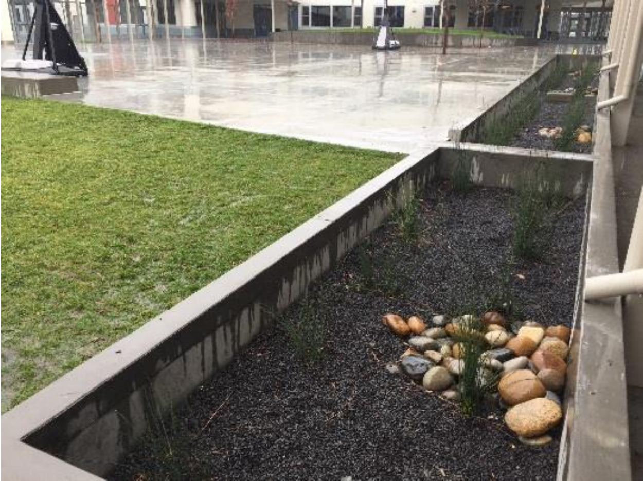
Figure 3-57. Rock cobbles under roof leader at school site in Emeryville. (Credit: EOA)
