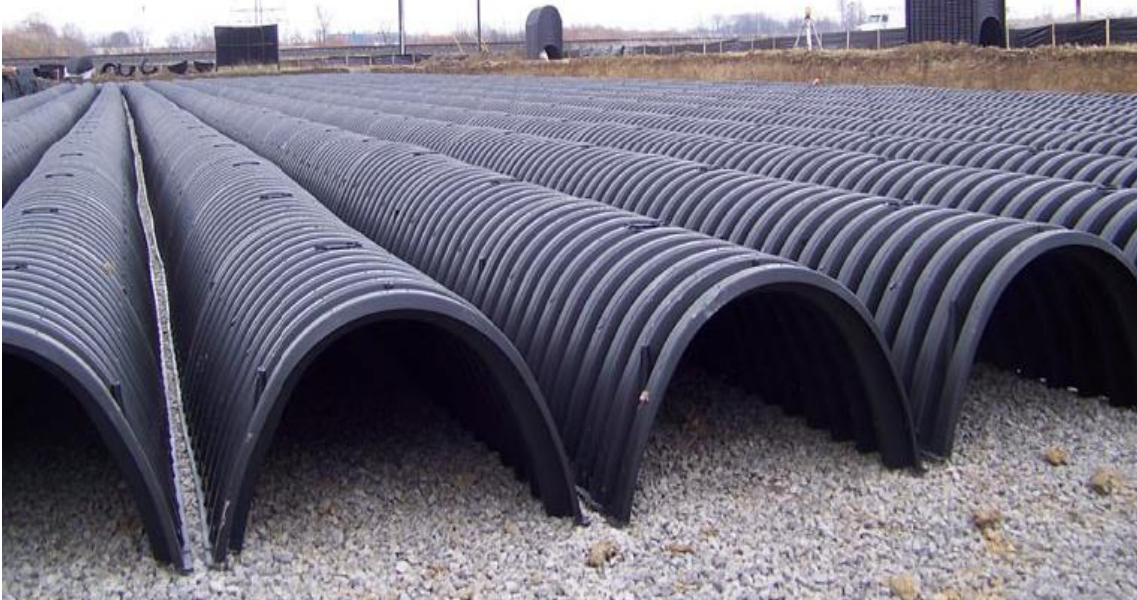
Figure 2-40. Photo of subsurface retention/infiltration system installation under a parking lot. (Credit: Contech)
