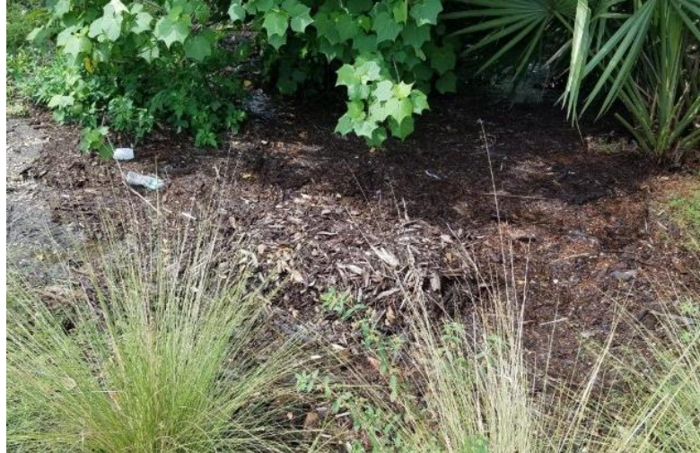
Figure 3-55. Mulch covering overflow drain. (Credit: City of San Jose)
