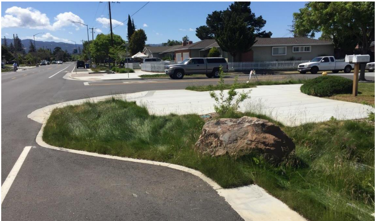
Figure 3-26. Partial stop-controlled T-intersection with flush curb, single-ramp, street-level crossing, and stormwater curb extension in Campbell (Credit: EOA)
