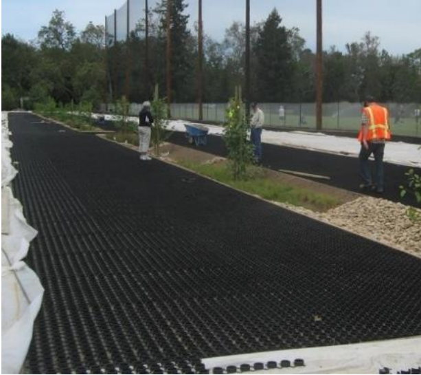
Figure 6-26. Parking bays contain recycled plastic geocells that support vehicle weight. Drain rock is below. (Credit: Cupertino)
