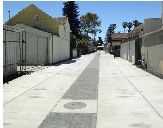
Figure 6-8. Pervious pavement over infiltration trench in Martha Gardens Alley. (Credit: San Jose)
