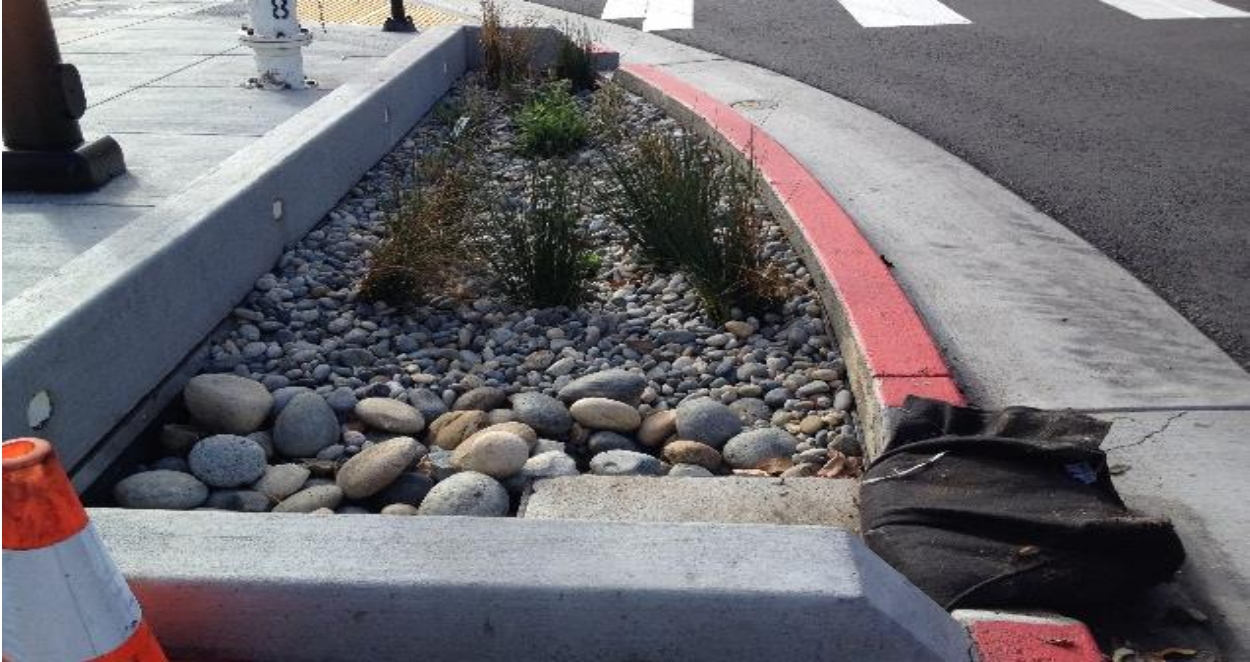
Figure 3-54. Rock and cobble mulch with temporary blockage of inlet during plant establishment in San Francisco. (Credit: EOA)
