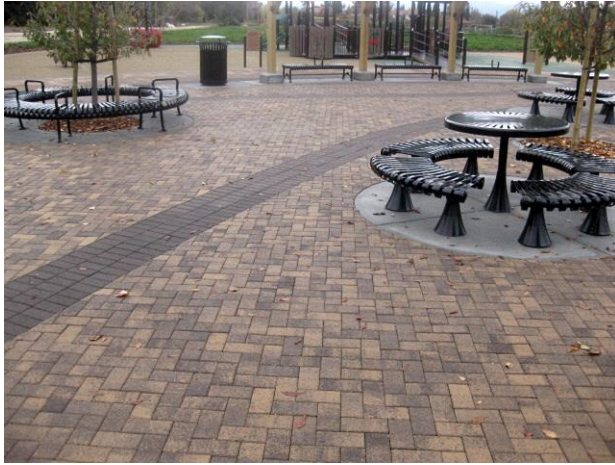
Figure 6-20. Close-up of permeable pavers in the plaza area. (Credit: San Jose)
