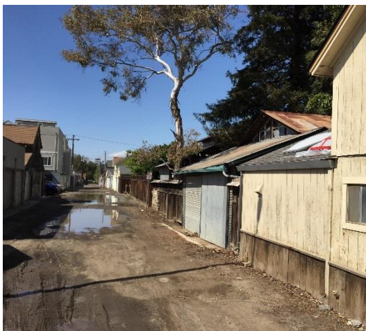
Figure 6-9. Unpaved surfaces & poor pavement prevented street sweeping and caused ponding in this area before project installation. (Credit: San Jose)
