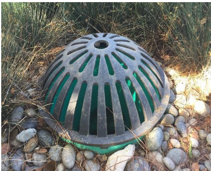
Figure 3-61. Beehive overflow riser cover in Union City. (Credit: EOA)
