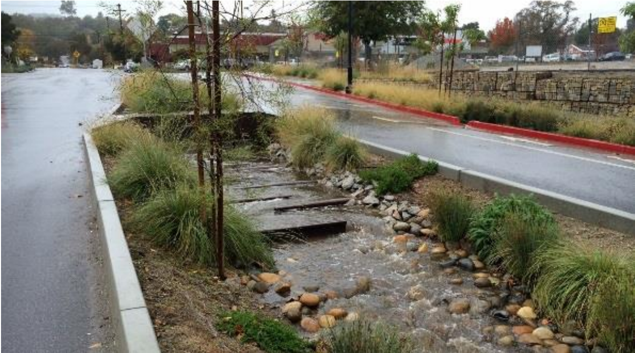
Figure 2-4. GSI measure in a depressed median in Paso Robles. (Credit: SvR Design and Cannon Engineering)
